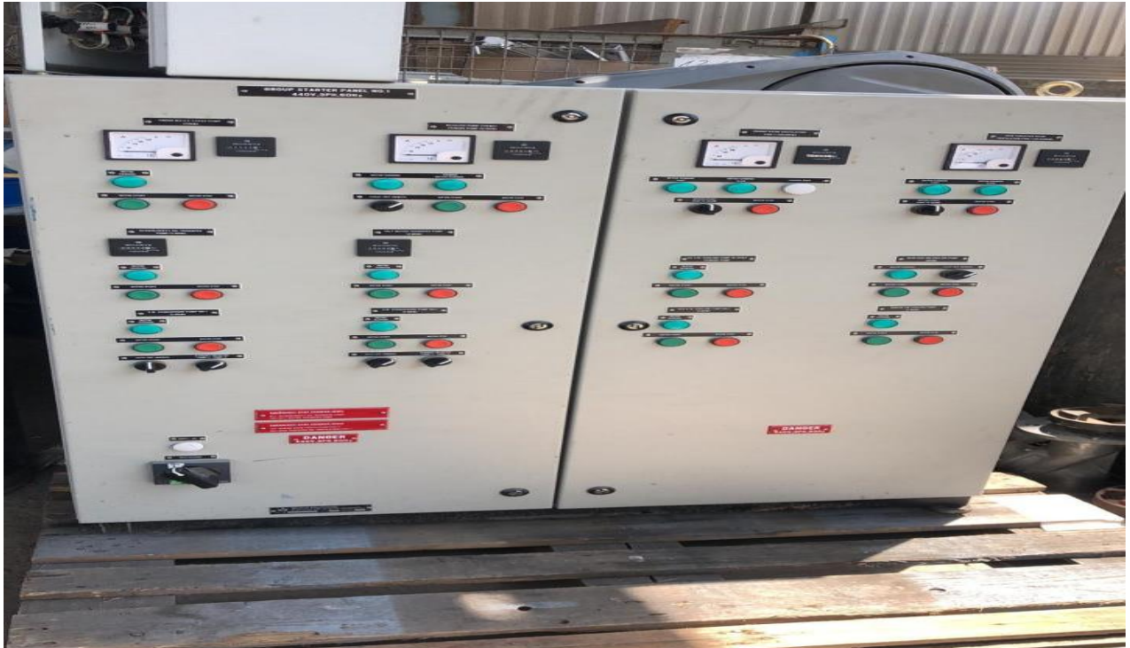
Power controls and automations
