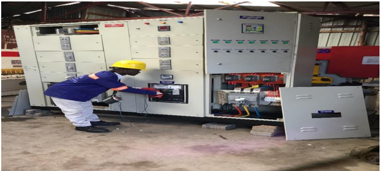
Power distribution board and accessories
