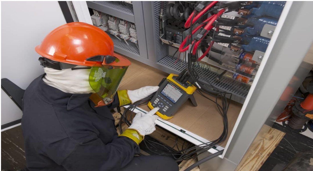
One of our employees carrying out power auditing
