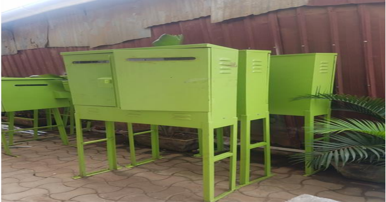
Electric panel enclosures and boxes
