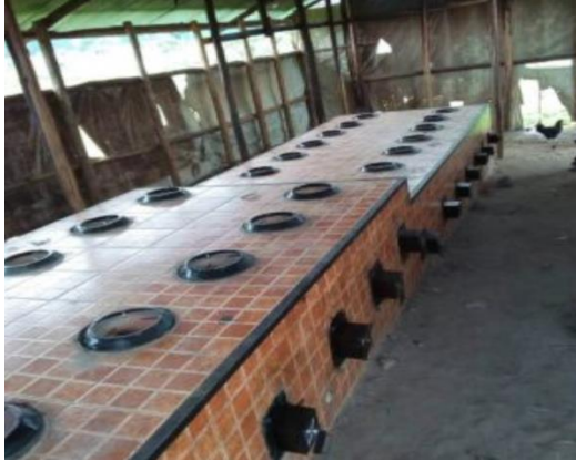
Institutional inbuilt burners
